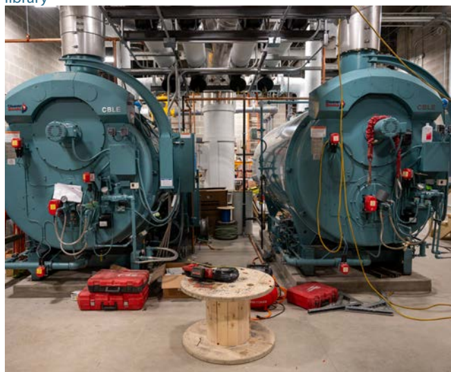
The Hospital's new Central Utility Plant will power our campus' future needs
